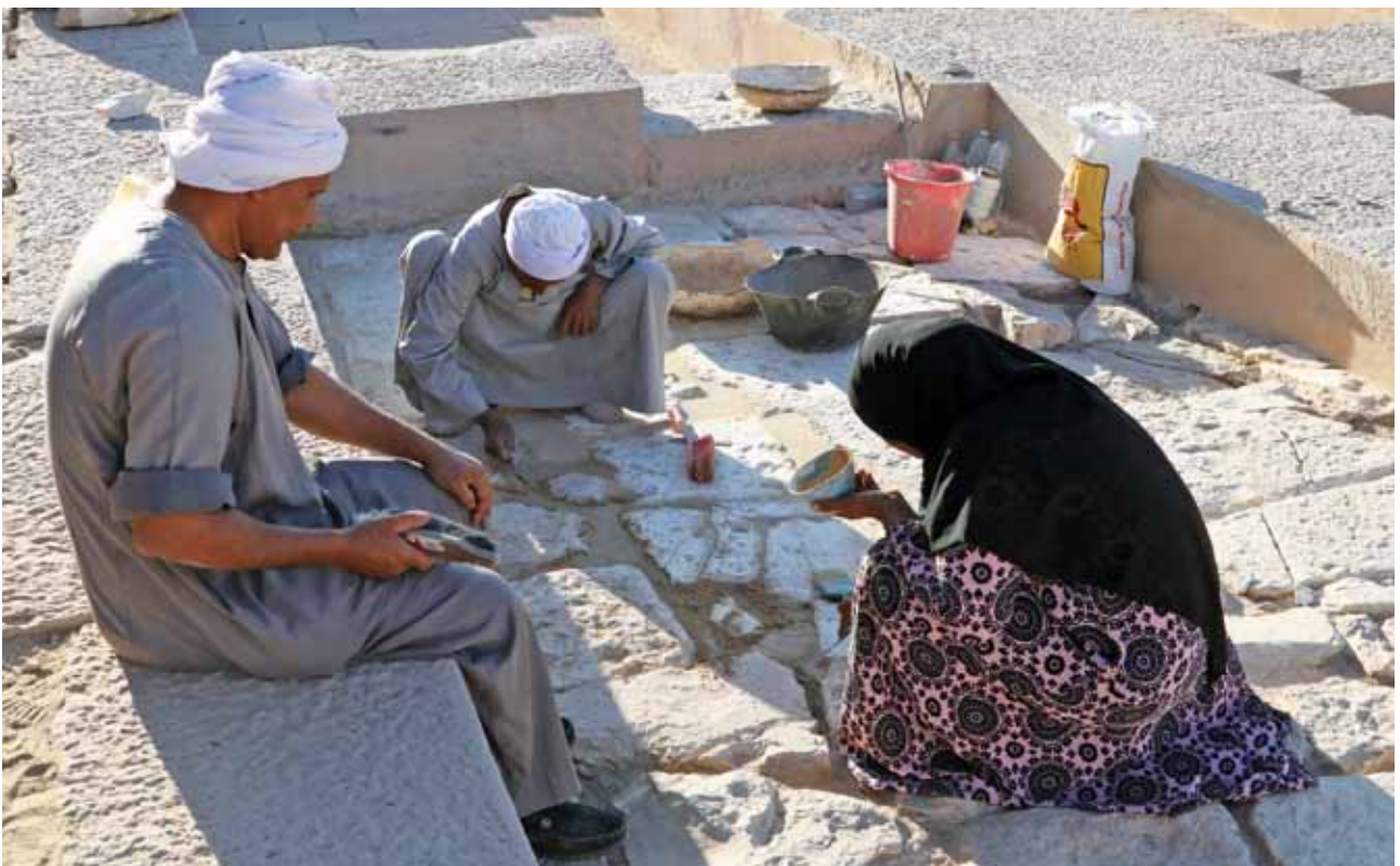
B.- RAMESSEUM. SECTOR BCS. Restoration of the floor tiles in the rooms of the south side of the temple. (Photo © Ahmed Abdel Hamid Ahmed).
