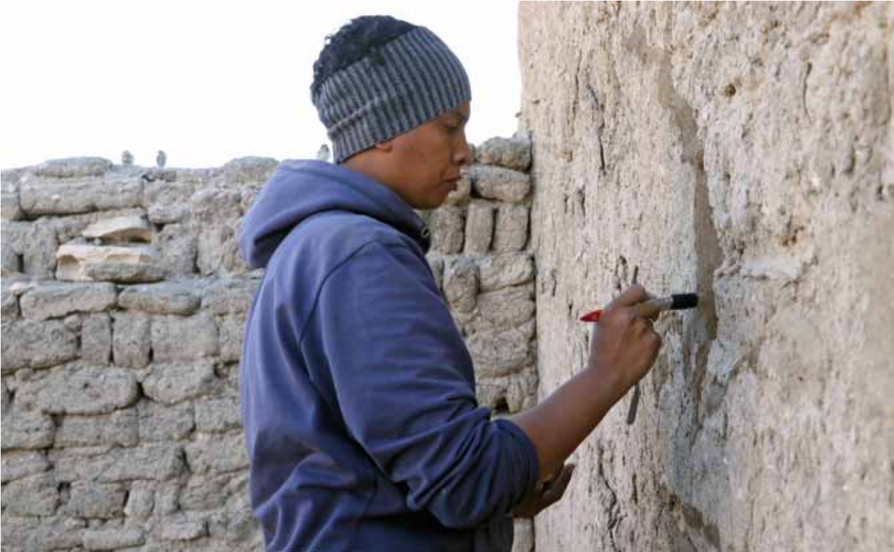
B.- RAMESSEUM. SECTOR STI.SA06. Consolidation of the ramesside wall coatings in room SA06. (Photo © Ahmed Abdel Hamid Ahmed).
