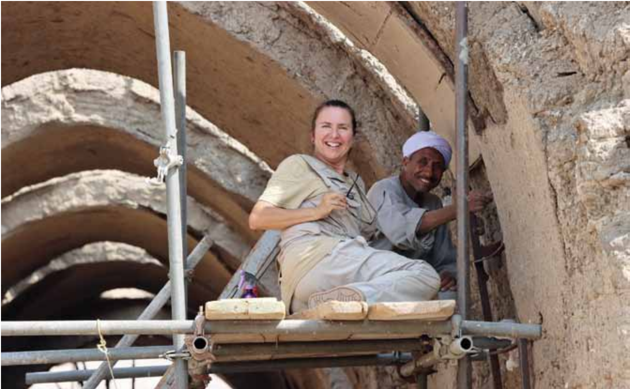
A.- STI sector. Work to consolidate a vault. (Photo Ossama Bassiouni El-Damanhoury/CEDAE).
