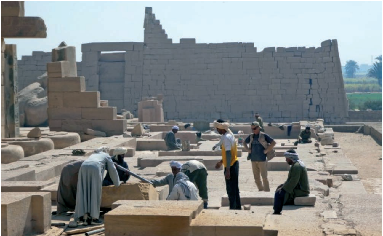
A.- Restoration work on the stone structures in the BCS sector (south side of the temple). (Photo Christian Leblanc).
